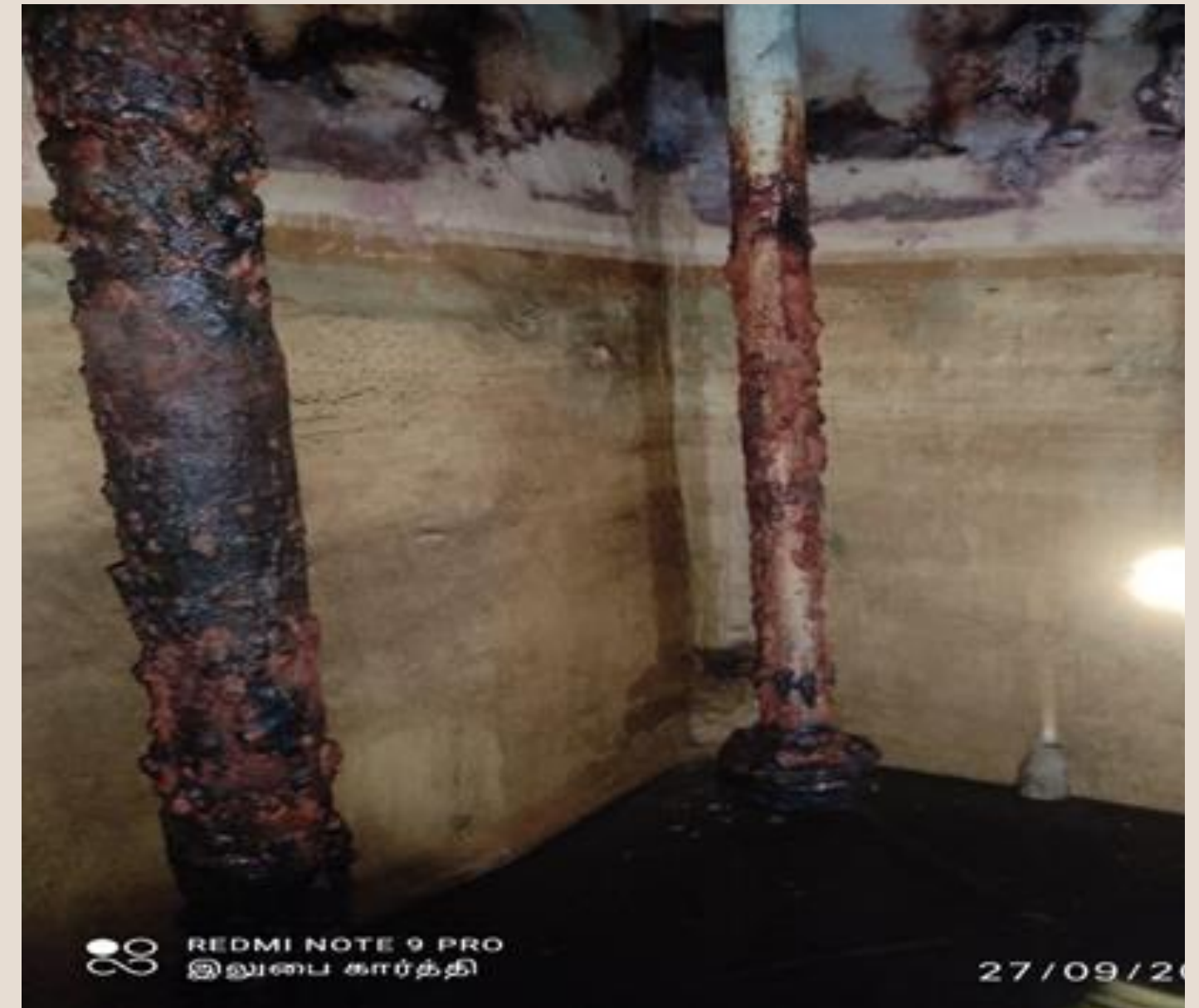
Overflow in sprinkler tank, severe corrosion detected in components and pipes
