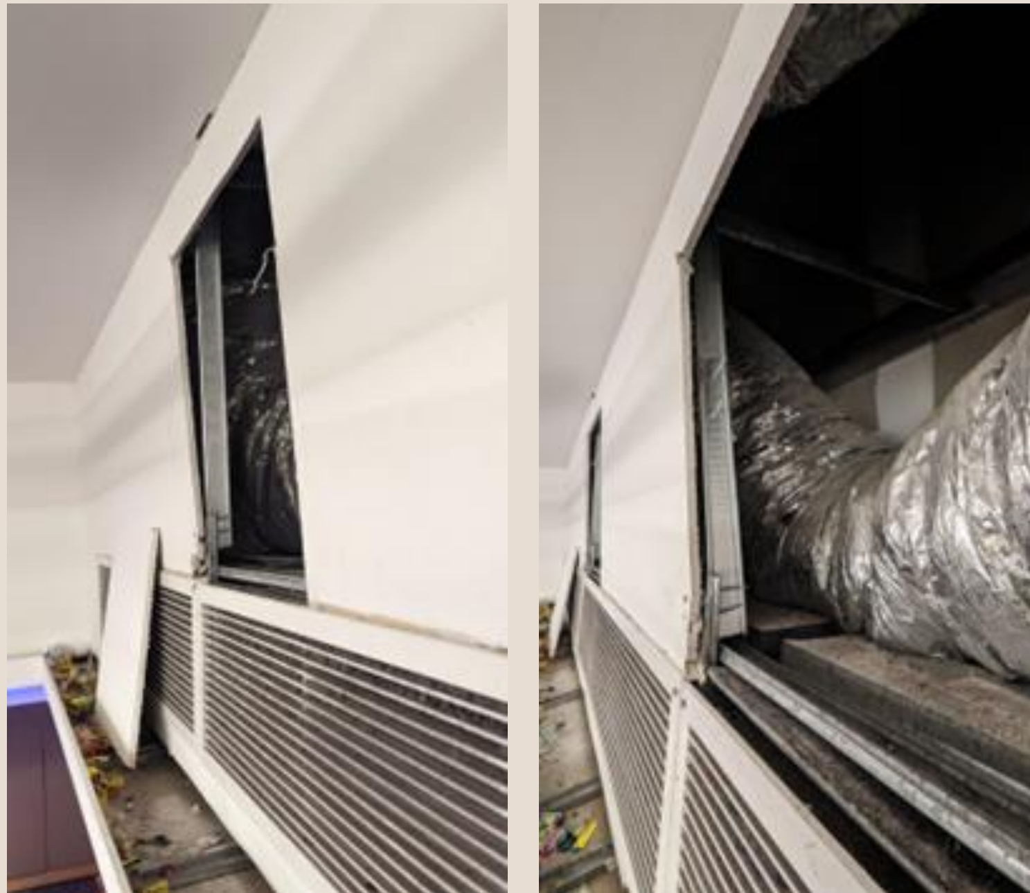
False ceiling at ballroom gave way
